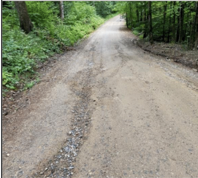
Erosion along Kaulback Road.
