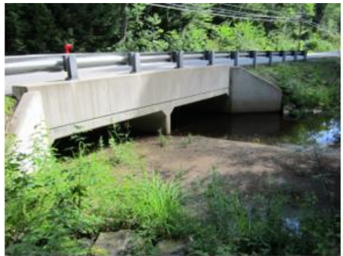
Sedimentation evident at a new box culvert along Black Brook at the Black Brook Rd crossing. Photo courtesy of Lang (2021).
